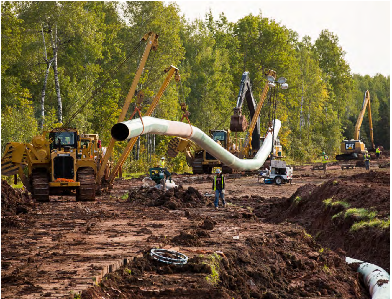
Construction vehicles install a portion of pipeline in the ground south of Superior, Wisconsin. (Derek Montgomery)
