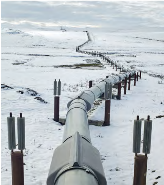
Oil pipeline surrounded by snow in Dalton Highway, Alaska. (Robert Valarcher)
