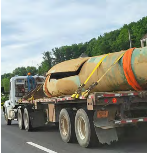
Photo of ruptured section of MVP pipe being hauled by a truck after a failed pressure testing. (Grace Terry)
